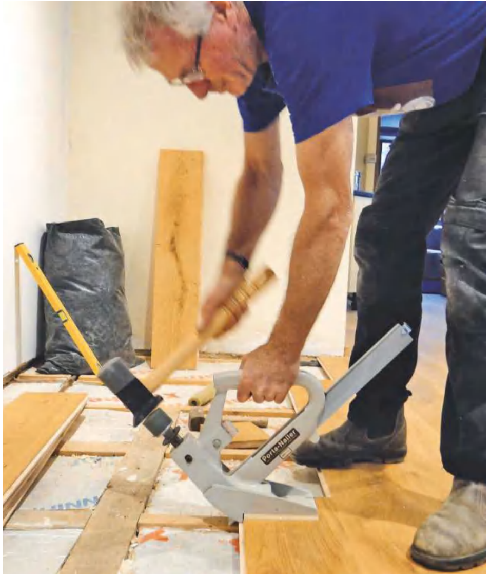
▲ Pic.2 Dickie laying the engineered flooring with the help of a nailing jig
